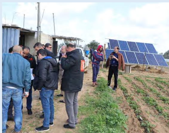
Photo: ©/ Fadi Harouda-PUI. Installation of photovoltaic systems for water pumping as a response to energy crisis in Gaza Strip.
